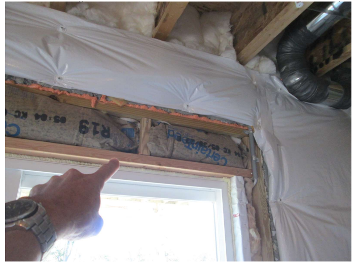
exposed paper facing poses fire hazard
