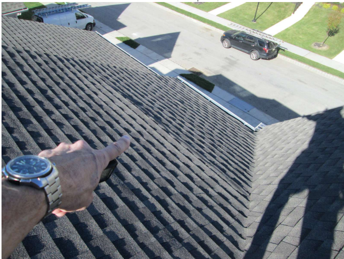
buckled shingles on front of main roof
