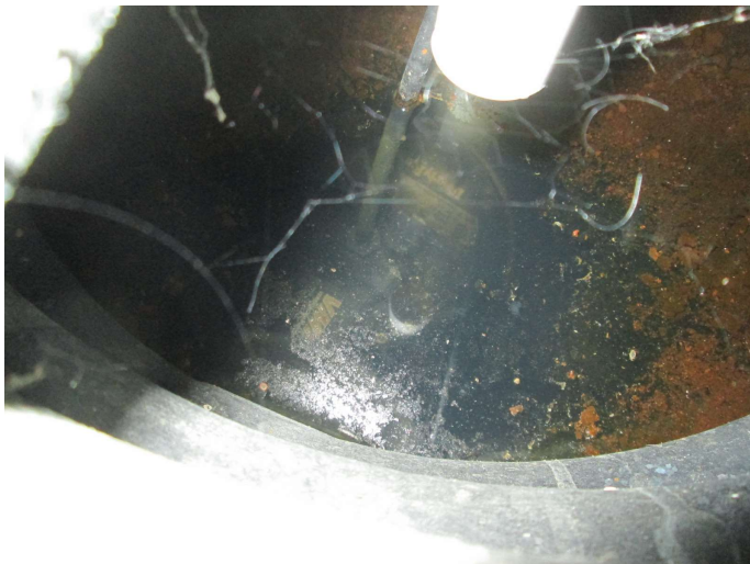
sump pump submerged in pit
