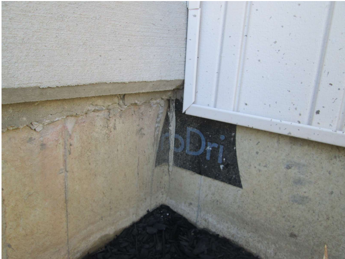
exposed house wrap
