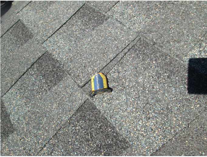
construction debris on roof
