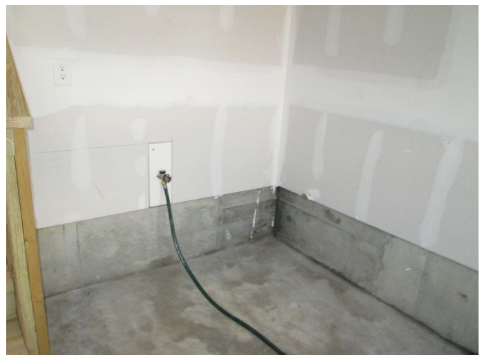
dampness inside garage
