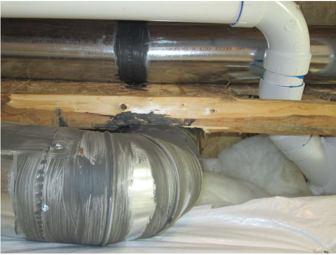
bottom chord of I-joist improperly notched
