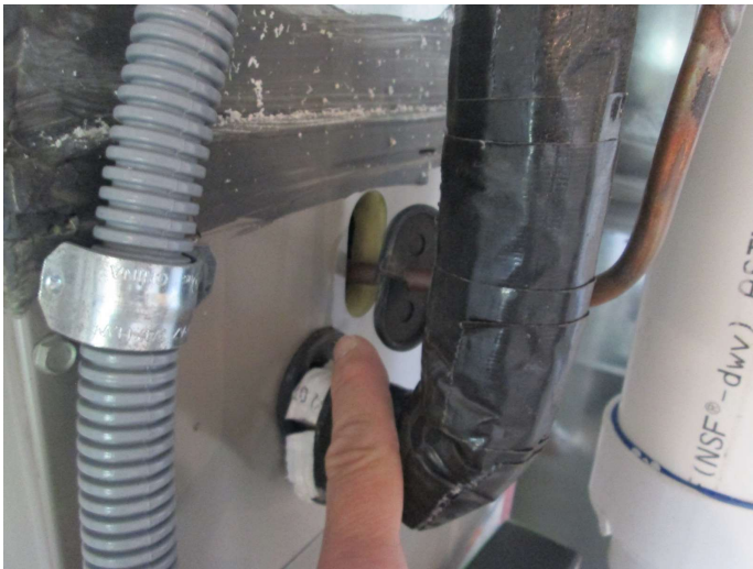
air leaks - grommet not secured
