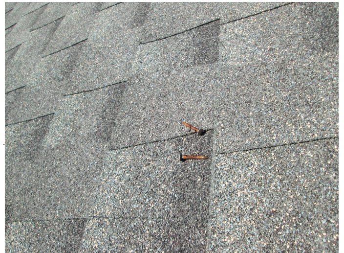
loose nails on roof
