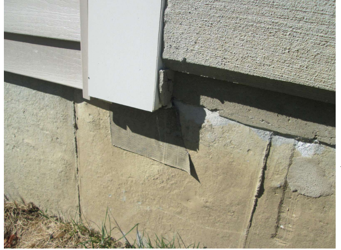
exposed house wrap
