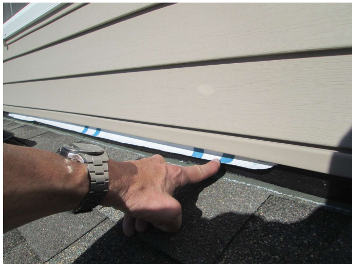
exposed house wrap
