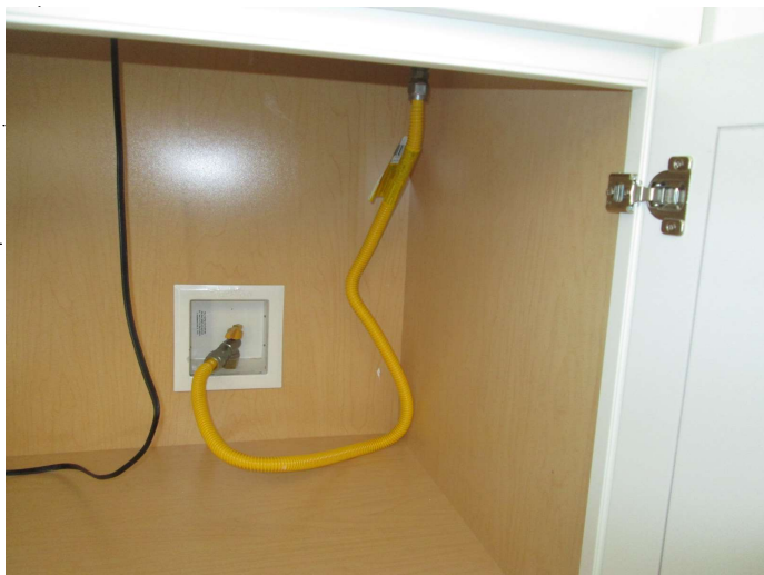
recommend having gas line secured up and off cabinet floor
