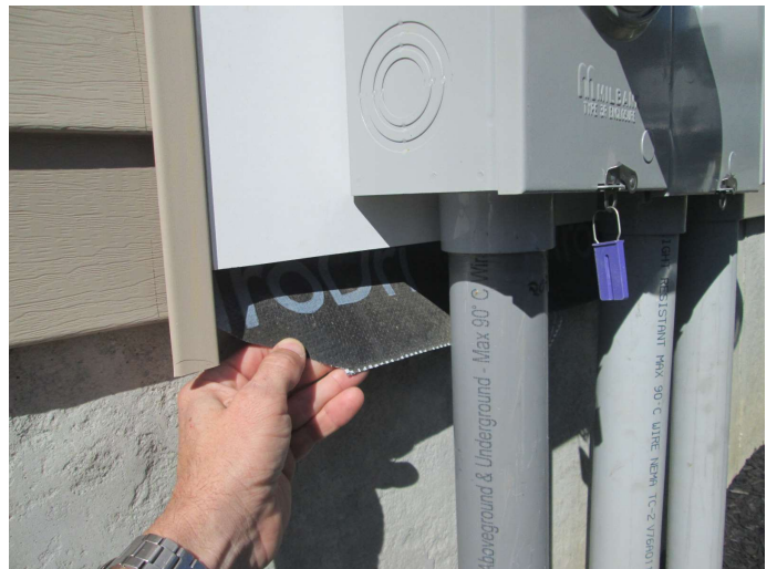
exposed house wrap
