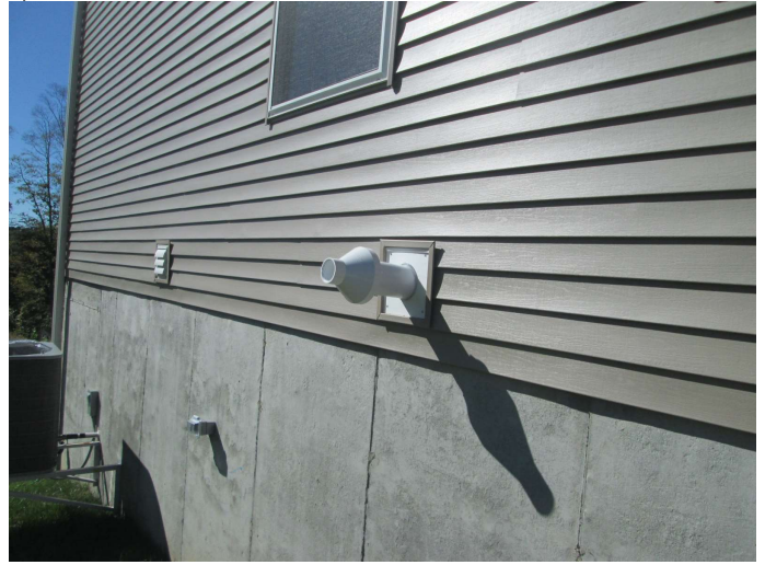
furnace vent pipe
