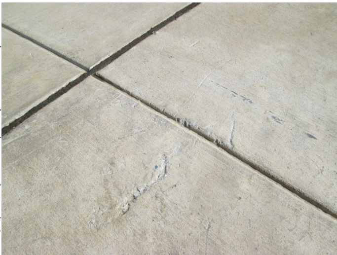
gouges on surface of sidewalk
