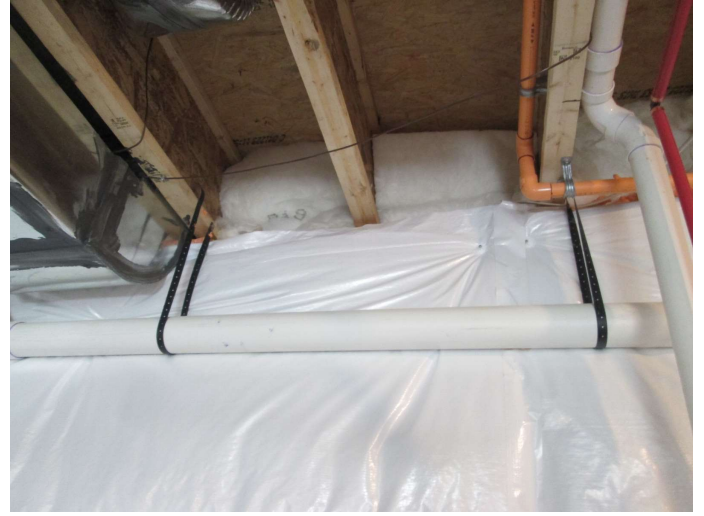
improper use of flexible vinyl straps to support drain line
