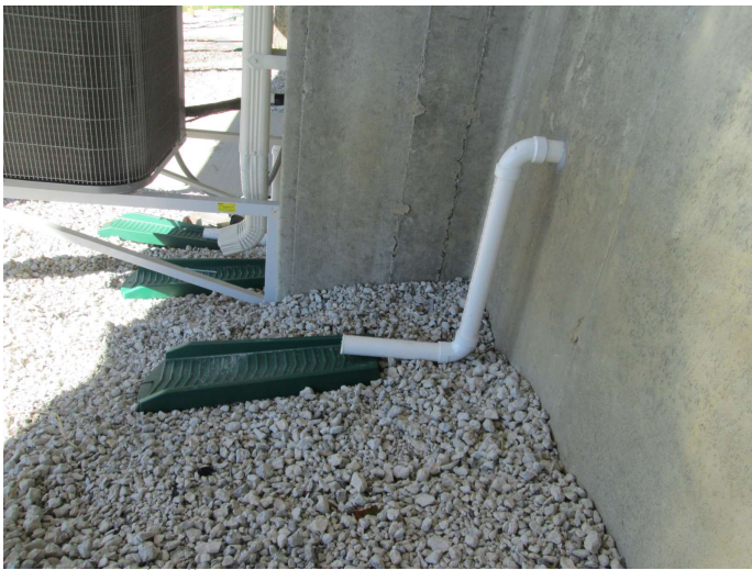
sump pump discharge pipe at rear exterior
