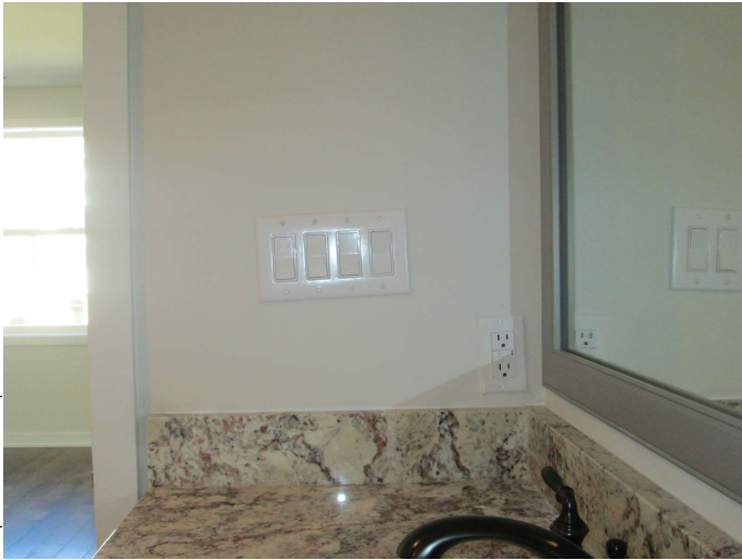
switches and outlet installed out of level
