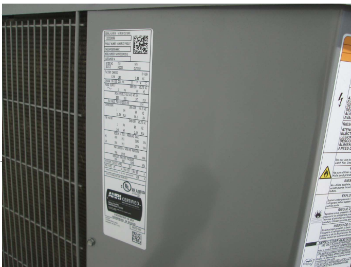
<1 year old 3 ton AC condenser
