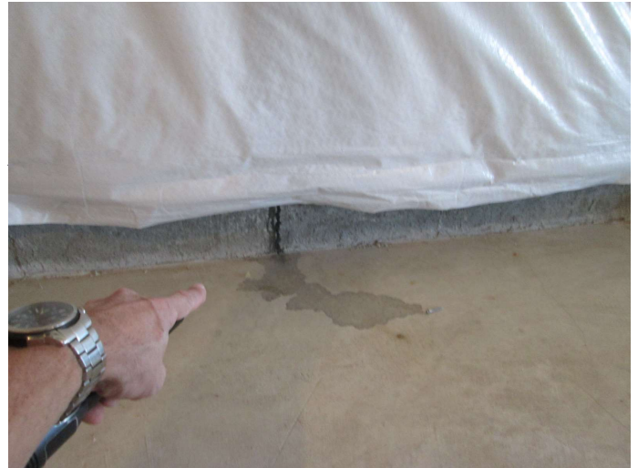
water penetration staining
