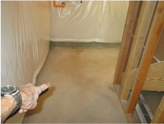
water penetration stain on floor
