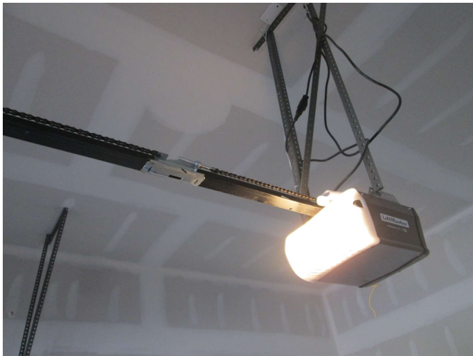
garage door disconnected from opener
