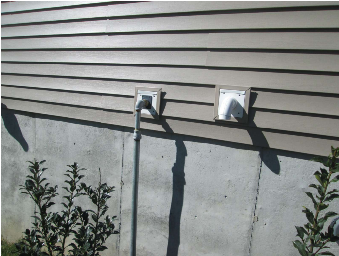
water heater vent pipe
