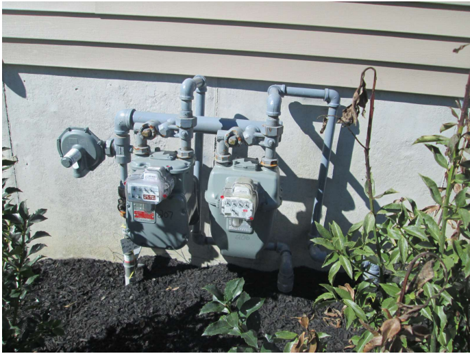
view of gas meters
