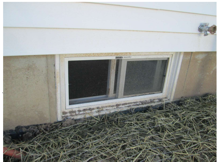
grades sloped towards house
