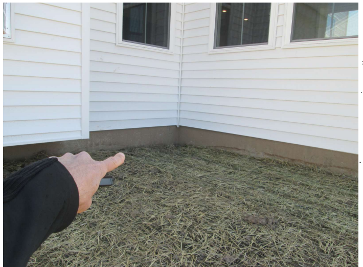
grades sloped towards house
