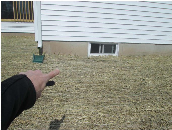
grades sloped towards house
