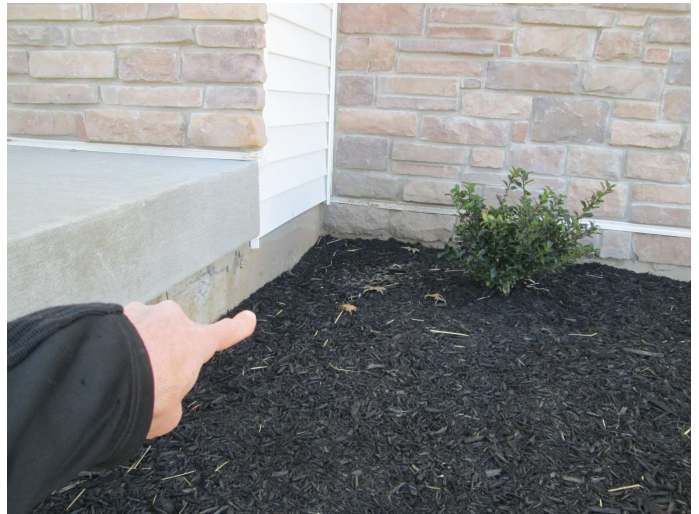
grades sloped towards house
