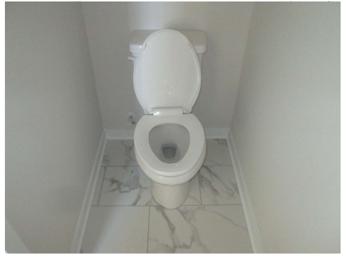
toilet not straight on floor
