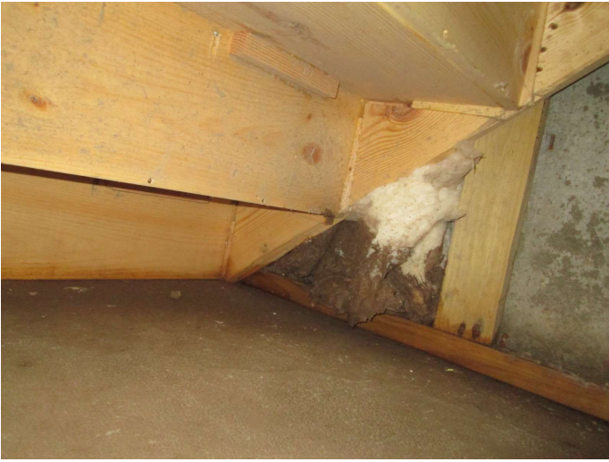
wet insulation beneath basement steps
