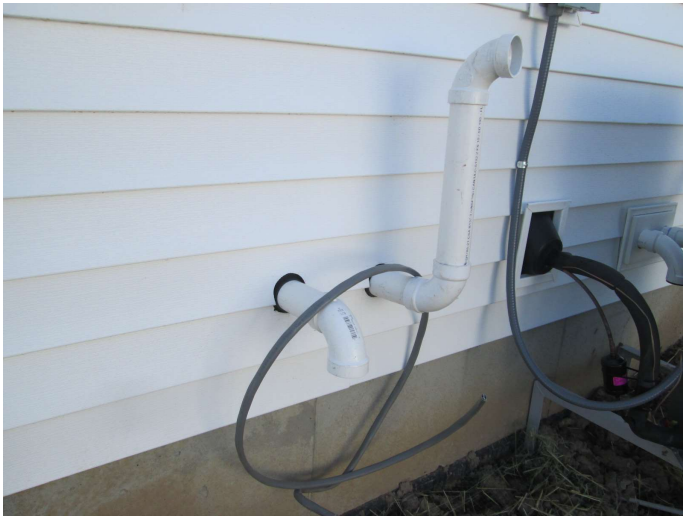
furnace vent pipes
