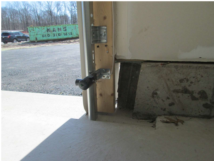
unsealed gap to exterior
