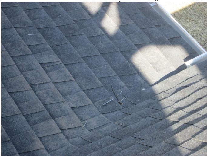
loose nails on roof
