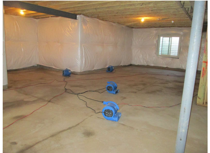
dampness on basement floor
