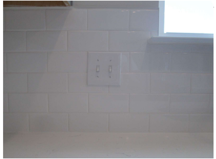
junction box out of level
