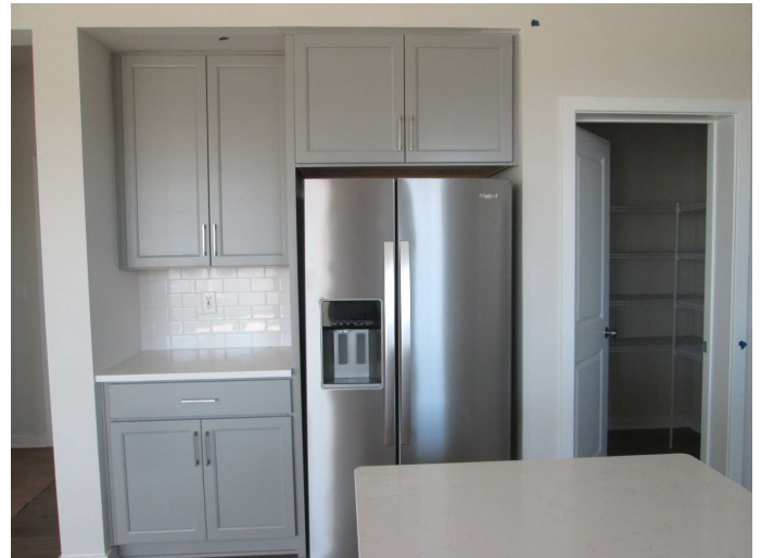
refrigerator not level on floor
