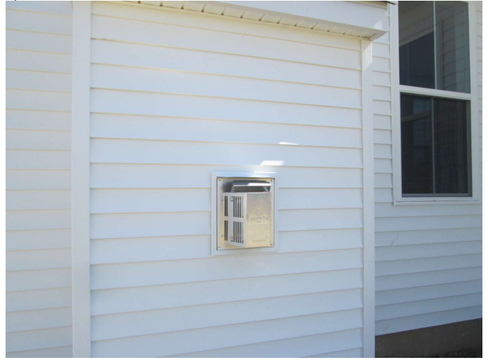
fireplace vent hood
