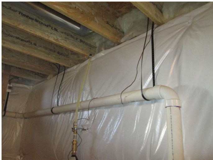
improper use of flexible vinyl straps - straps loose and not support
