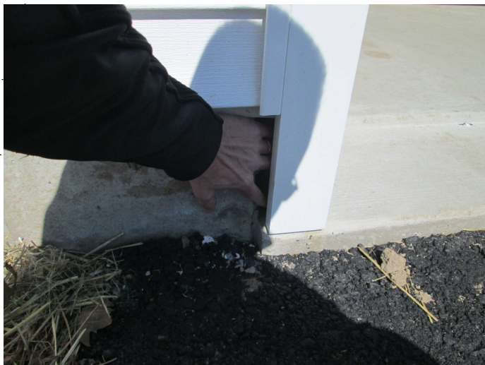
unsealed gaps at garage door frame
