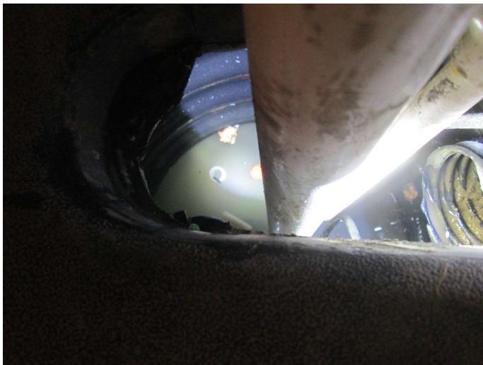
construction debris in sump pit
