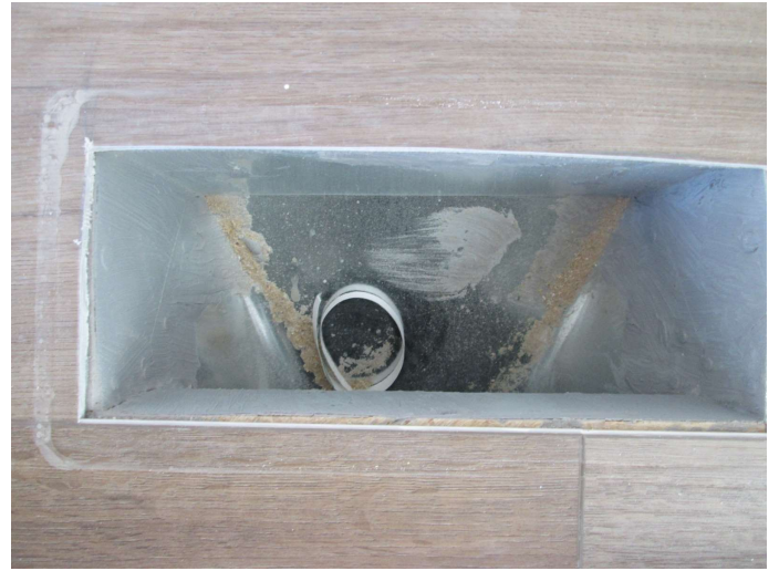
construction debris inside floor levels HVAC ducts
