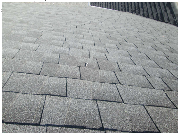
loose nails on roof
