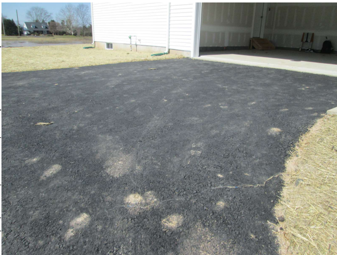
driveway installation incomplete
