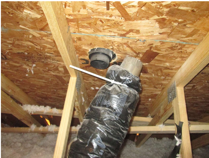
dryer exhaust duct disconnected in attic
