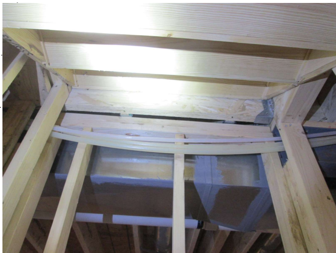
unsupported water supply lines
