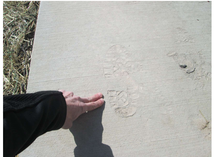
boot marks on walkway surface
