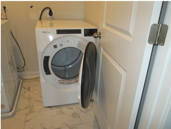
door to clothes dryer hits against entry door to laundry room
