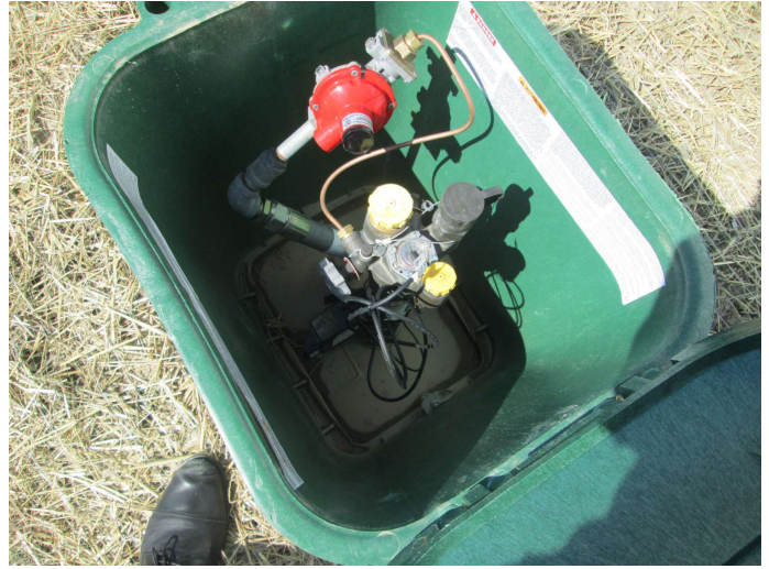
view of tank gauge
