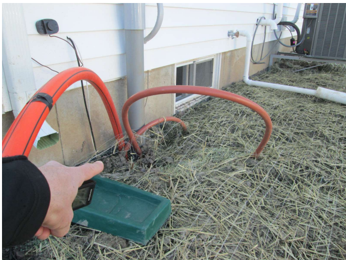
grades sloped towards house
