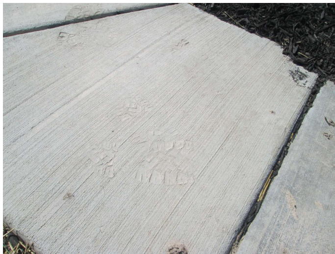
boot marks on walkway surface
