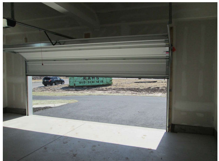
garage door automatic opener will not close door
