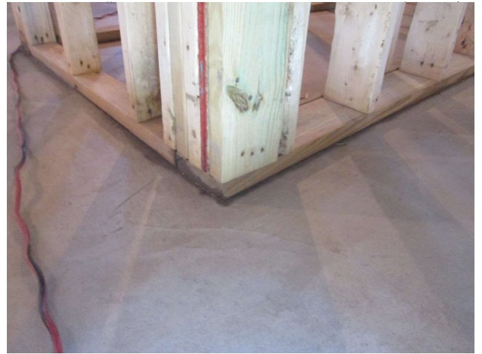
dampness on basement floor
