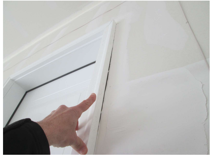
unsealed gaps around door frame inside garage
