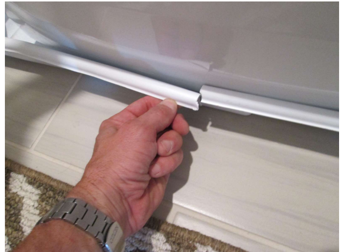
washing machine overflow pan cracked
