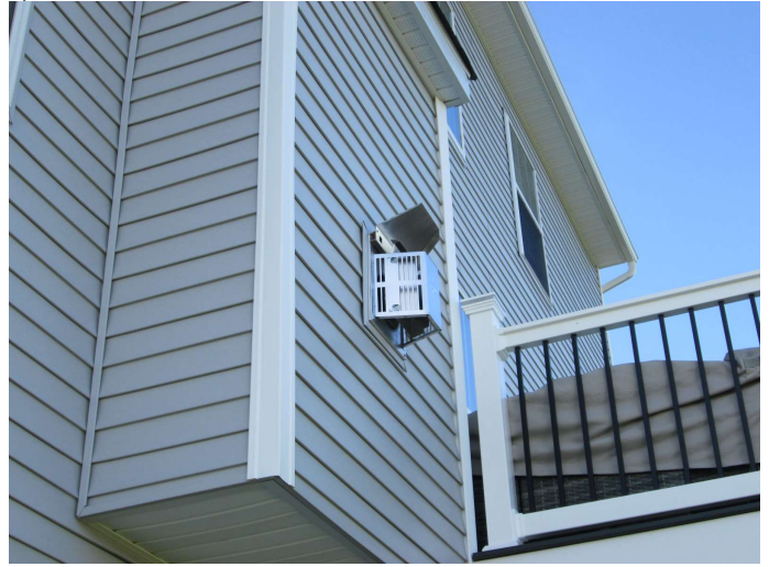
fireplace vent hood
