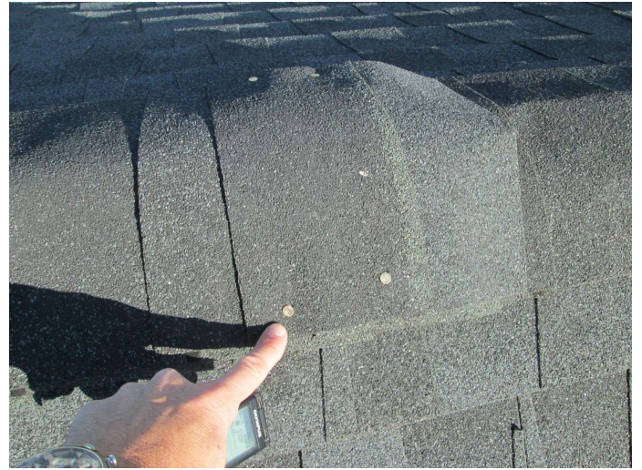
exposed unsealed nail heads on roof surfaces
