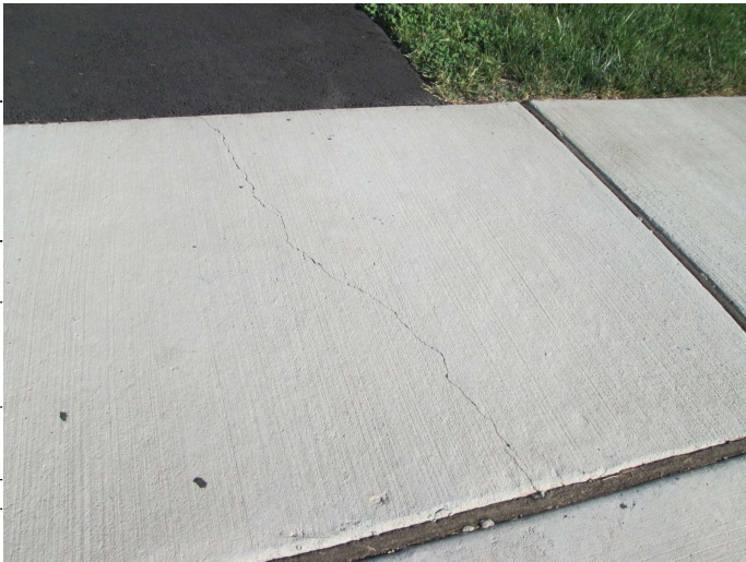
crack on sidewalk slab
