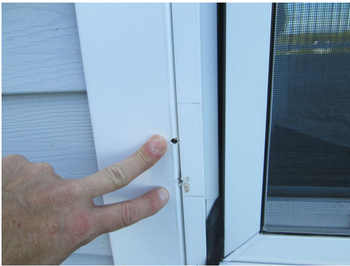
holes in trim capping
