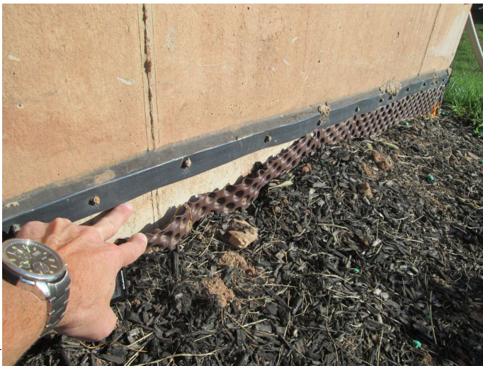
foundation membrane separated
