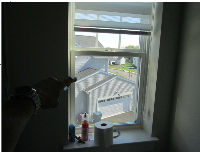
bathroom window difficult to open and close
