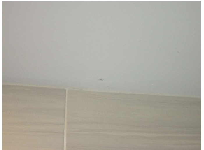
exposed screw heads on ceiling above shower stall
