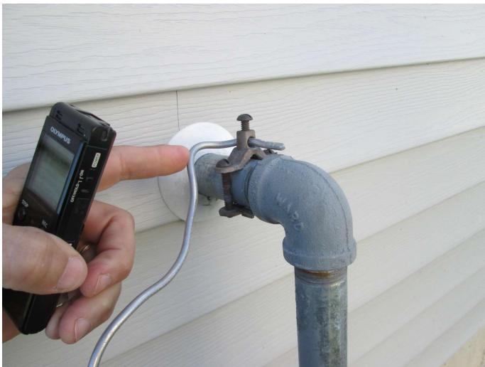
bonding conductor not secured
