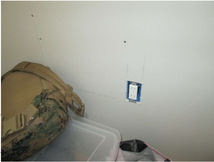
multiple coverplates missing
