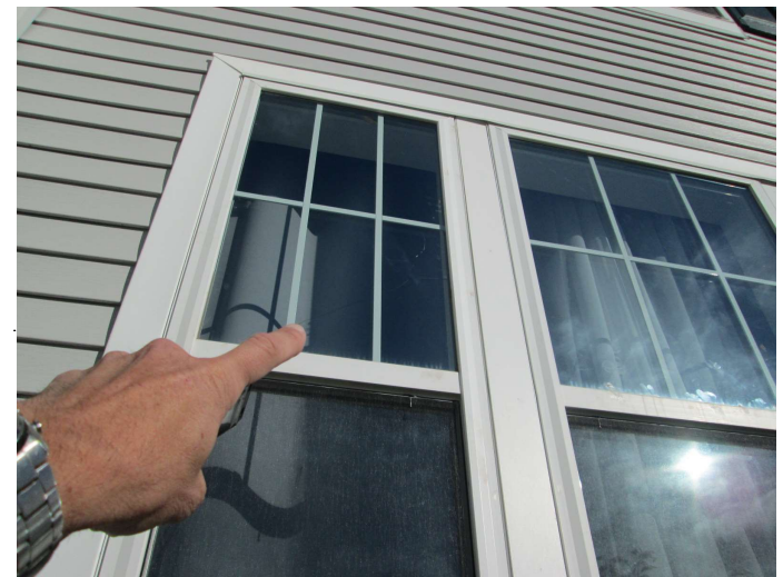
broken pane on front office window
