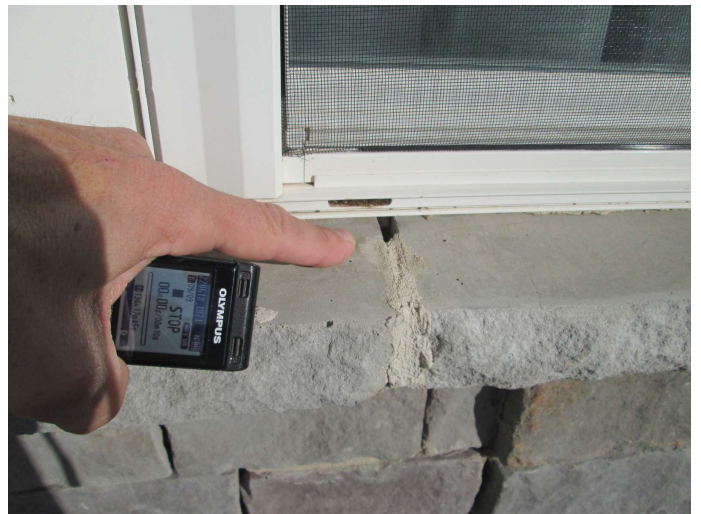
voids in pointing
