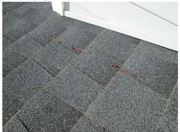
loose nails and debris on roof
