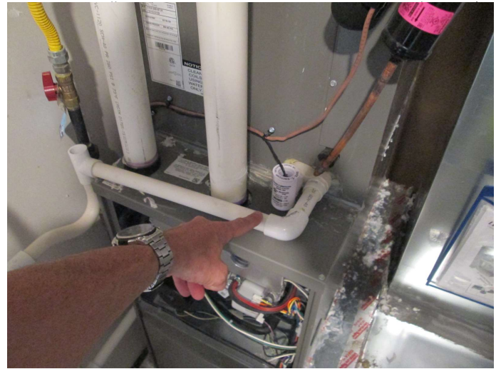
air leaks on zone #2 furnace cabinet
