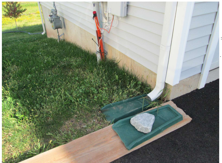
downspouts exhausting too close to foundation
