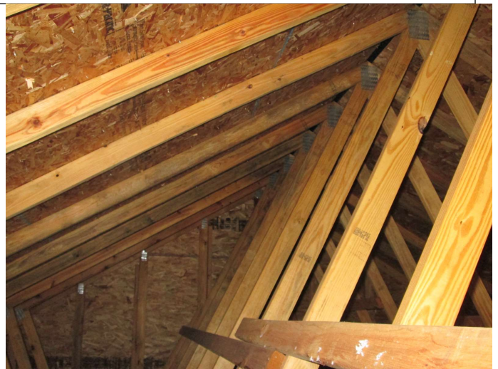
mold on trusses in attic
