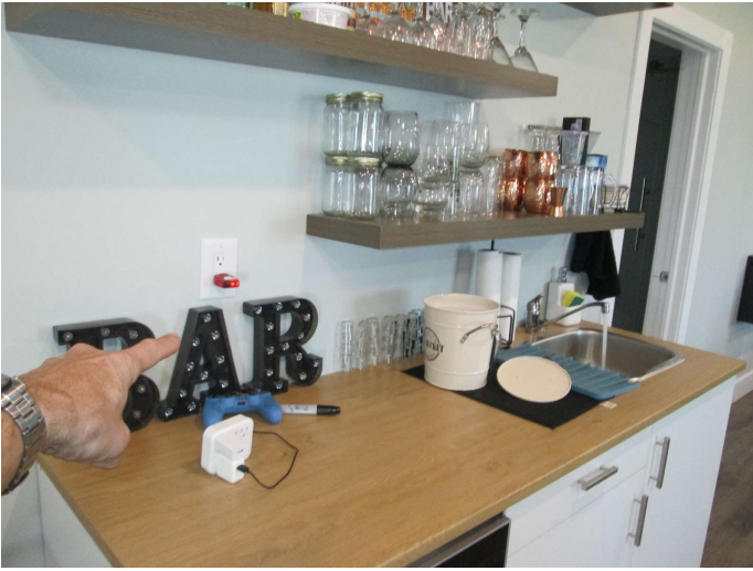
outlet above wet bar not GFI
