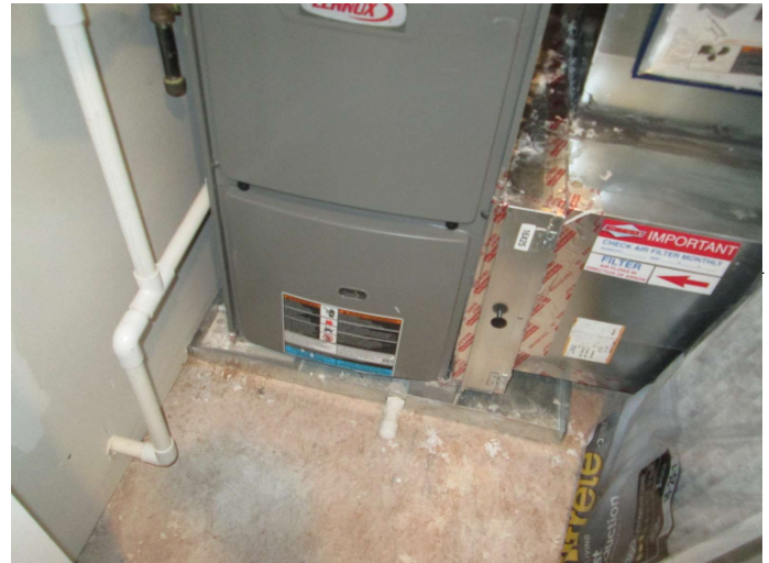
overflow pans beneath furnaces have no drain lines & no water sensing shut offs
