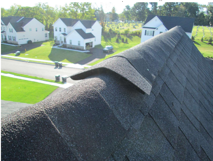
ridge vent end and shingles not properly secured
