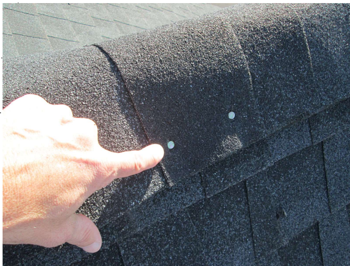
exposed unsealed nail heads on roof surfaces
