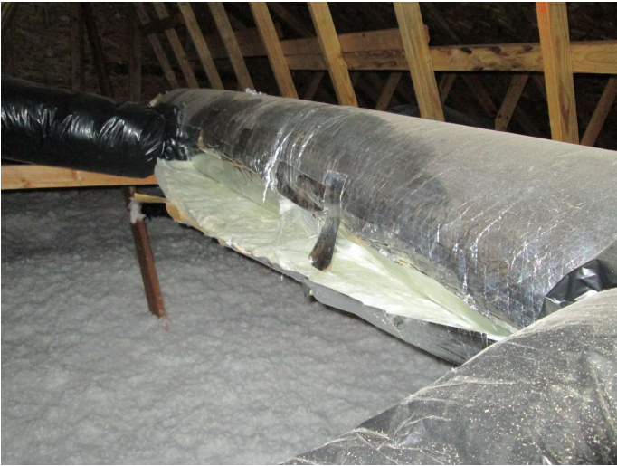
unsecured insulation on duct in attic
