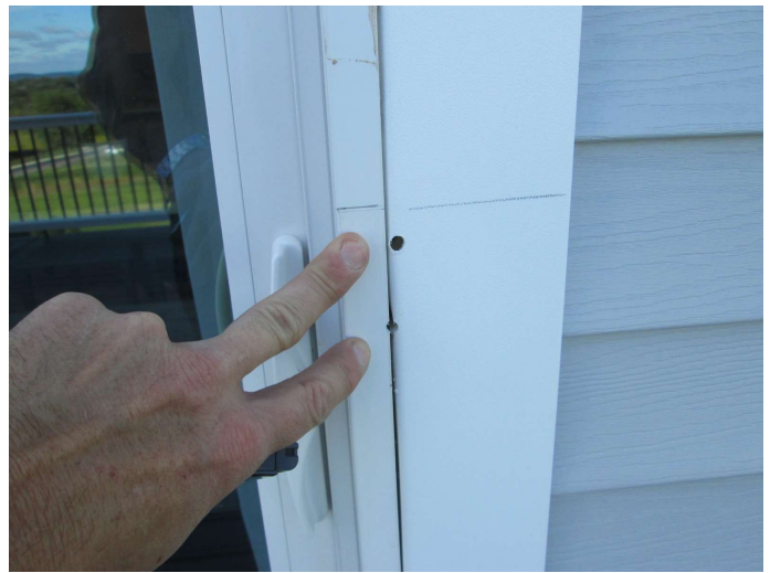
holes in trim capping
