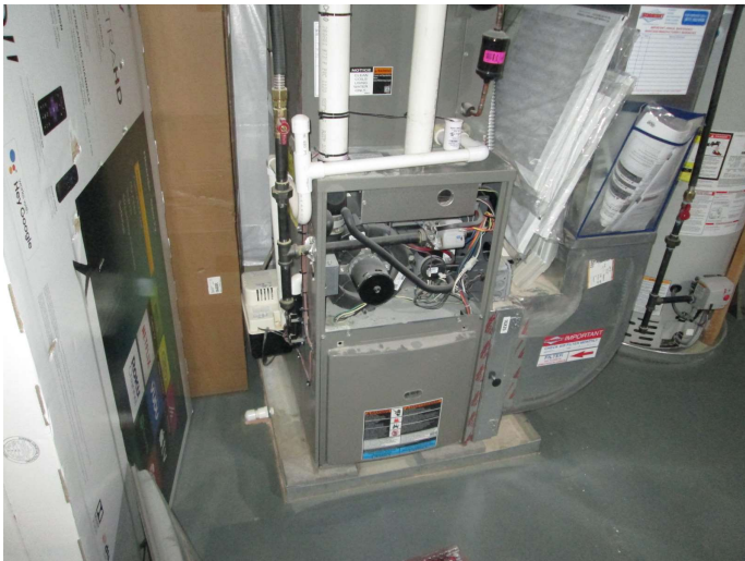
overflow pans beneath furnaces have no drain lines & no water sensing shut offs
