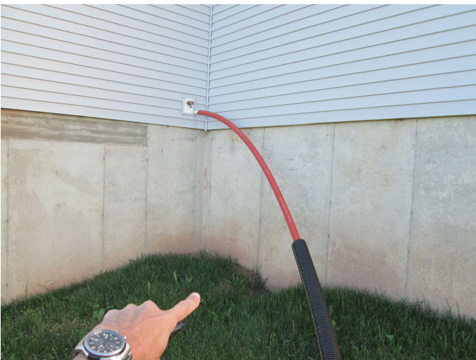
washout of grade beneath sump pump pipe
