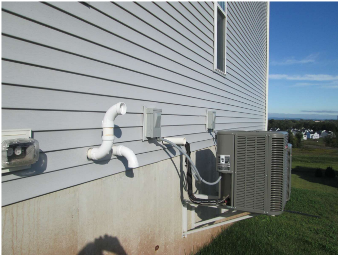
furnace and water heater vent pipes
