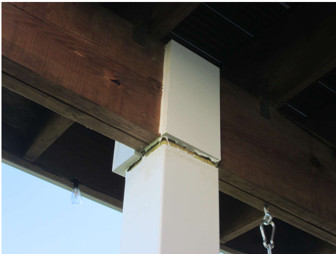
separated caulk seal at top of vinyl sleeve on deck post
