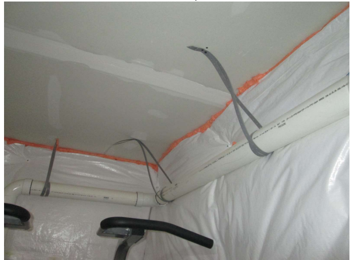
improper / inadequate strapping support on drain lines
